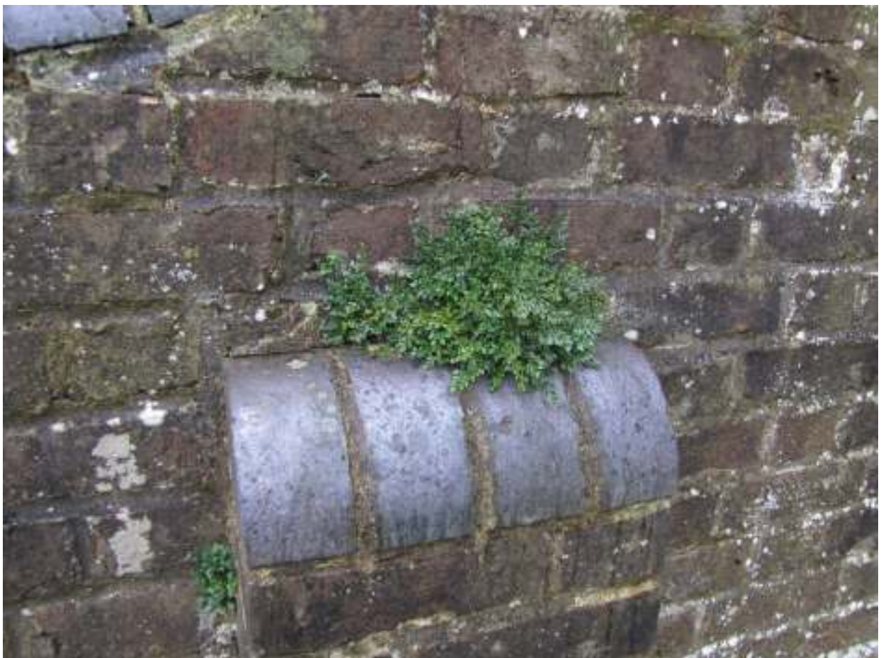
P4 – Part of the boundary wall with Wall Rue and lichens
