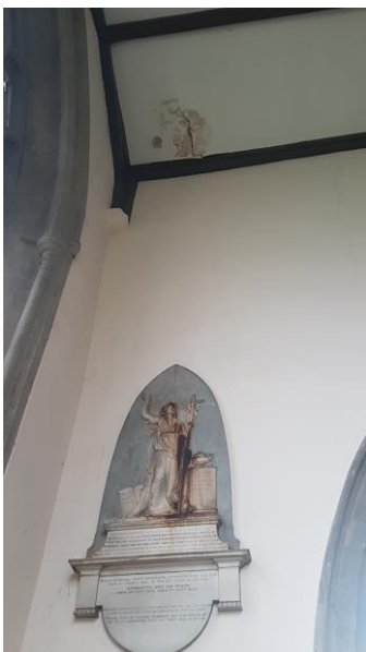
Damage to the roof in the Lady Chapel in St Peter's caused by leaks in the roof.
