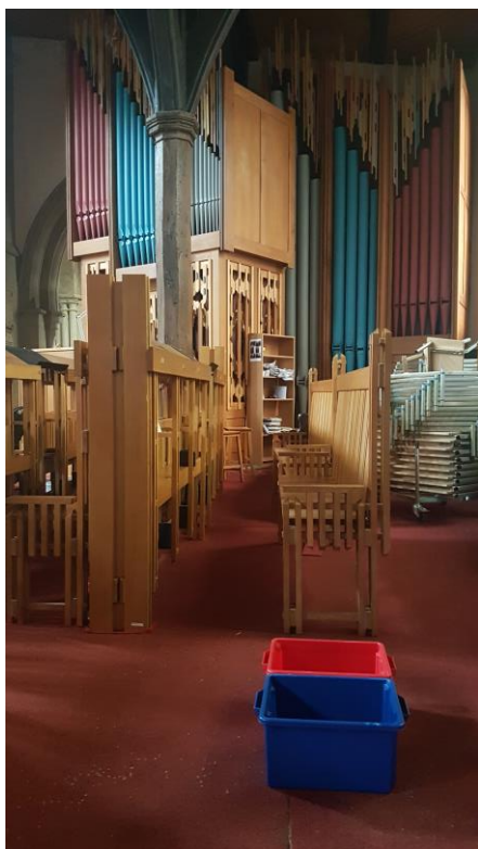
Buckets collect the water from leaks in the roof of St John's Chantry
