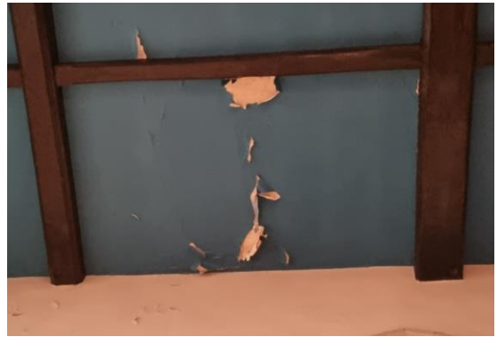
Damage in St Catherine's Chapel
