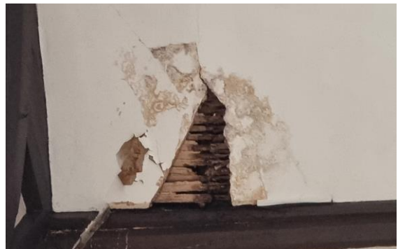
Damage in the North Transept
